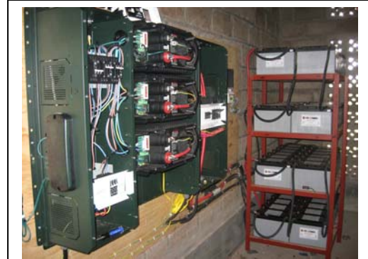
Inverters and Battery Rack
